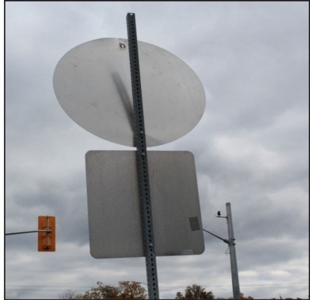
New, no heavy truck sign. The top fastener on the “new” sign has failed. Planning is required to determine whether the sign fasteners should be replaced or if the “new” portion of the sign can be removed.
